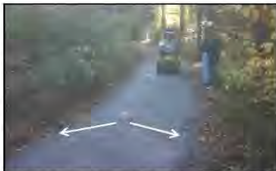
TSA can be successfully placed with small equipment for short sections of trail. Proper compaction at optimum moisture is crucial. Note the crown in the finished surface.
